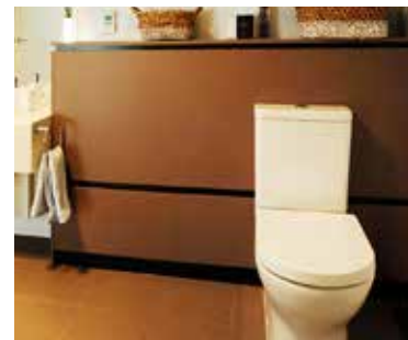
A false wall behind the toilet allows for concealment of pipes to the toilet, including additional piping, should the toilet need to be relocated in future, Hunter Housing Project.
