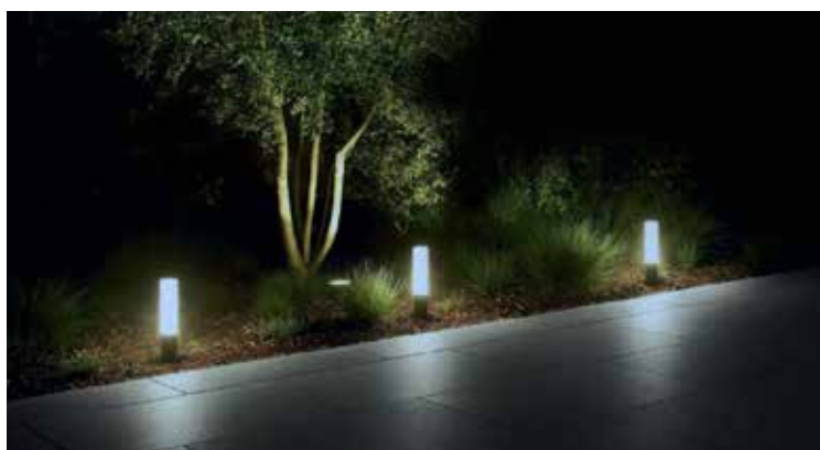
External entry lighting.
