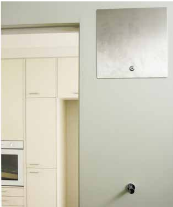
Access panel for thermostatic mixing valve, Mission Australia (Victoria) housing, MSN Architects.
